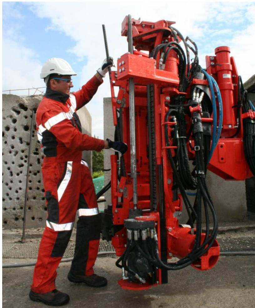
Figure 5-New TULPM bolting turret
