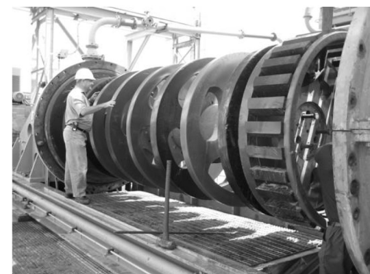
Figure 10: Photographs of the M 10 000 mill internals, showing the damaged discs and the discs after replacement following one of the internal failure incidents
